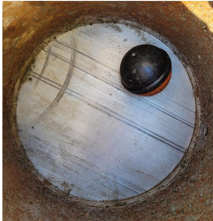
Figure 1 A photograph showing a Piper instrument cluster inside a 200 mm diameter pipe
