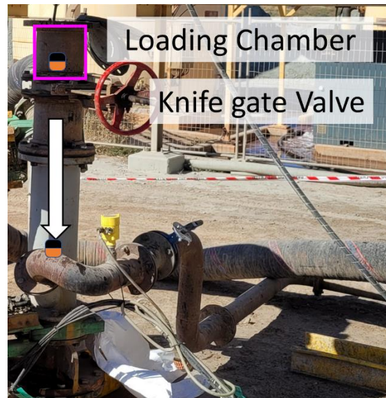
Figure 2 A photograph showing the knife gate valve spool for launching the Piper into the UDS
